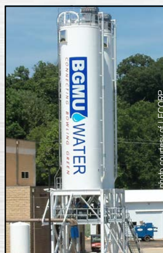
Truck load-out system designed by LECORP, Paducah, KY for BGMU Water.
