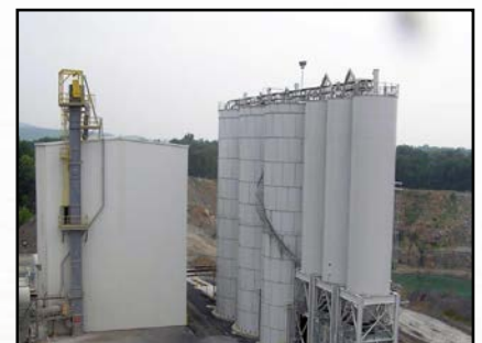
(3) 400 ton tanks added to an existing 5000 ton CST bolted tank facility. 1200 addition tons added in 8 weeks from order to delivery.
