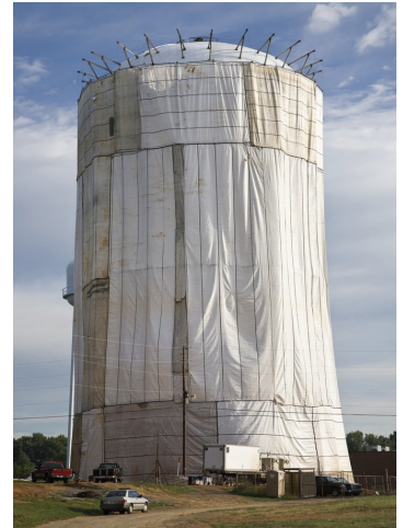
Figure 2 – Covering a field-welded tank for control of particulate in and out of the application area
