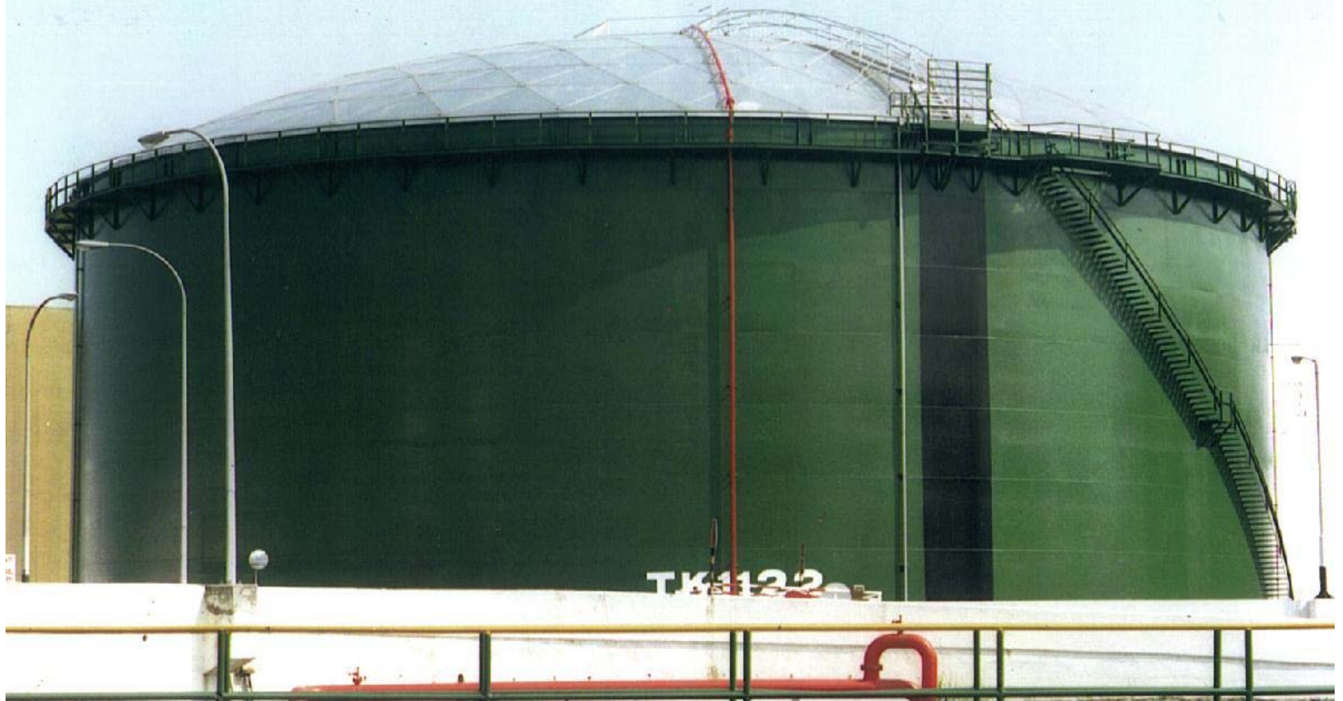
Esso Singapore 45.4m Fuel Oil Storage Tank; conversion from steel cone roof to aluminum dome; completed January, 1997.
